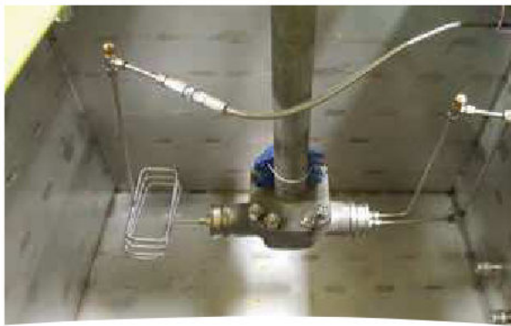
2" McCANNA CryoSeal test preparation
